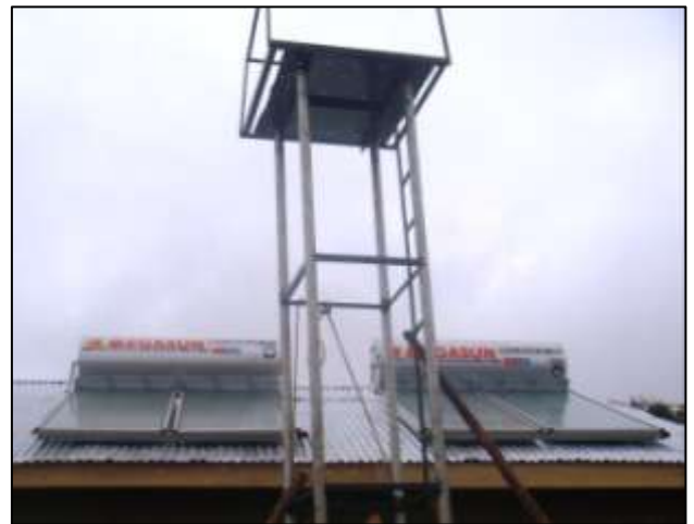
Two 300-litre solar water heaters were installed on the rooftop at Peace School in July. A pump feeds harvested rainwater to an elevated tank, which then flows to the heaters. The elevated tank was not yet been installed when this picture was taken.
